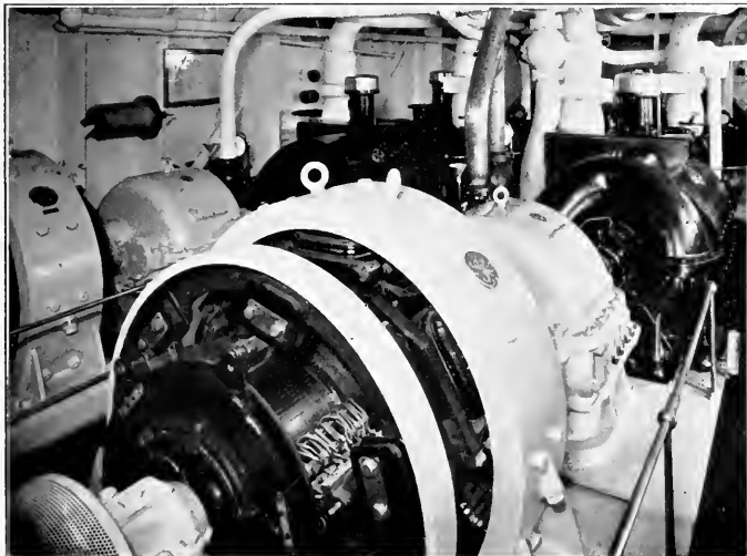
On the generator flat of the Steamship President Hoover's engine room are installed four General-Electric 500-kilowatt turbo-generating sets.
